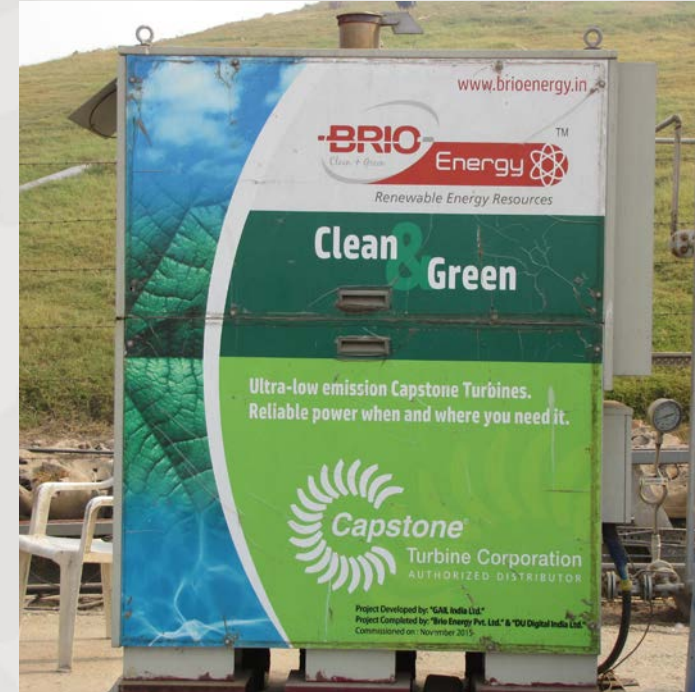
Microturbine at East Delhi landfill
